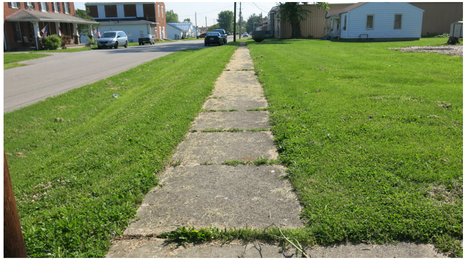
Figure 2. Example of poor (top) and fair (bottom) walkability conditions that could benefit from maintenance and further contextual considerations such as street tree planting and shade
